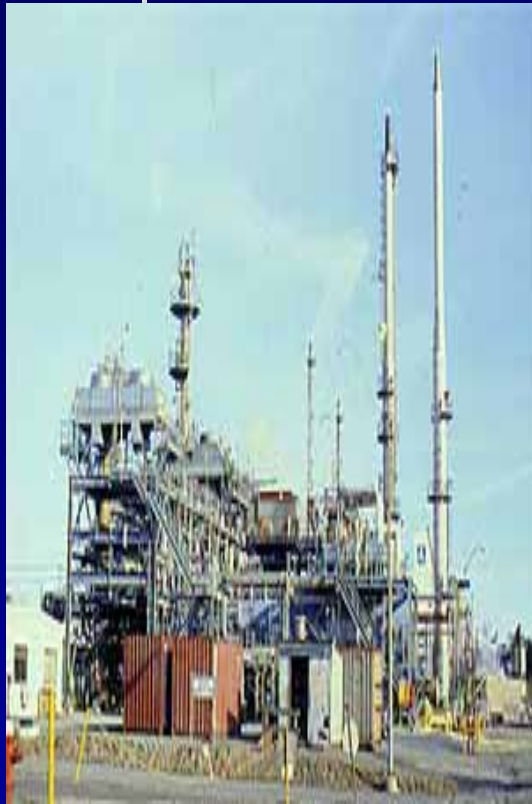
Sulfur Recovery Unit
